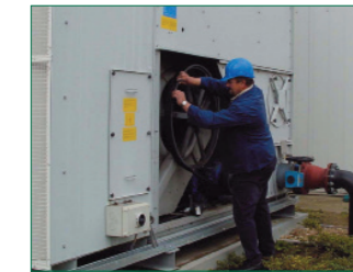
Easily accessible fan drive system at ground level
