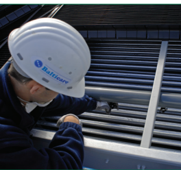
Full access to spray distribution system
