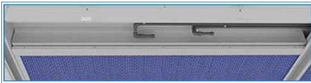
Pre-cooler water distribution
