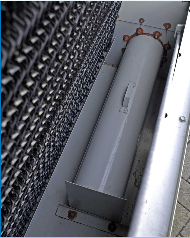
Cold water basin and basin strainer
